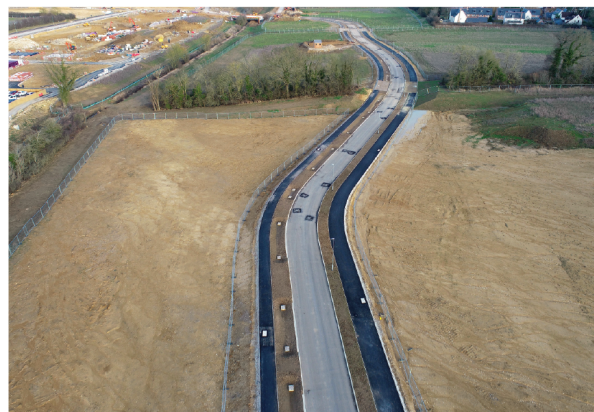
Good progress is being made on remaining infrastructure such as the roads, footpaths and accompanying work.
